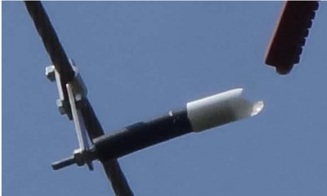
Fig 8: Broken indicator of Arrester on pole #6 of sub-branch
