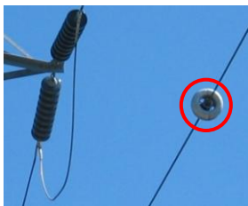
Fig. 8. Power Donut TM installed in a transmission line.
