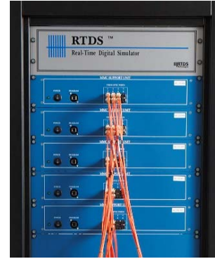
Figure 7. Fiber optic cable connection between MMC valve FPGAs and control FPGAs.
