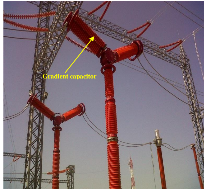
Fig. 5 400 kV breaker in Choacahui substation
